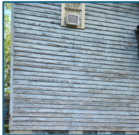
Wood Siding – Needs Repair
